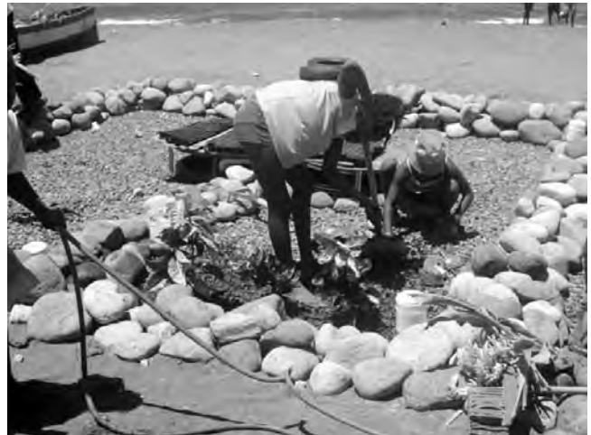
Local school children have selected salt tolerant plants and planted them into the beach level wetland that is now treating sewage and wastewater from communal showers.
