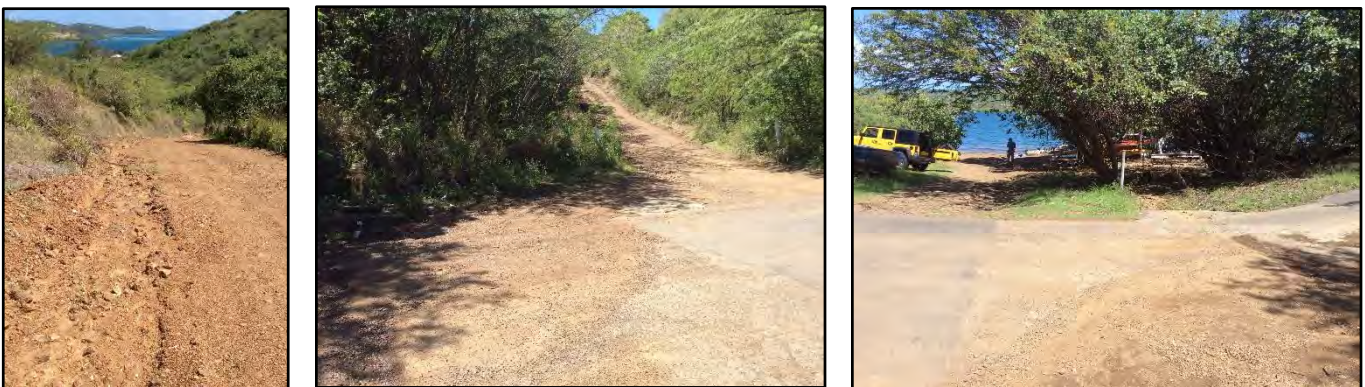
Figure 5. Example actual unstable dirt roads in Culebra.
