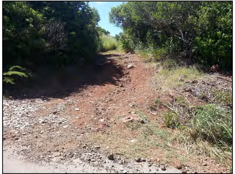
Figure 12. Dirt road prior stabilization.
