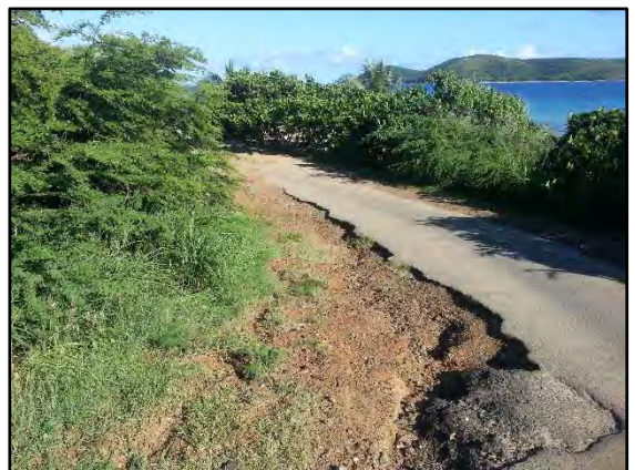
Figure 10. Undesirable watercourses prior stabilization.
