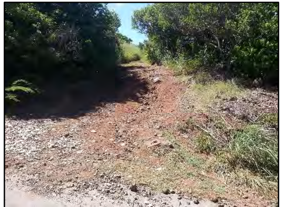
Figure 9. Dirt road prior stabilization.
