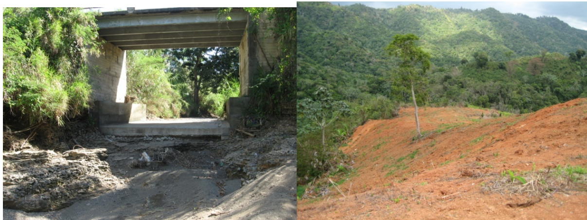
Figure 6. Left: Rio Loco river culvert, completely dry in April 2008; Right: Example of typical land clearing in upper watershed for coffee cultivation, without soil stabilization.
