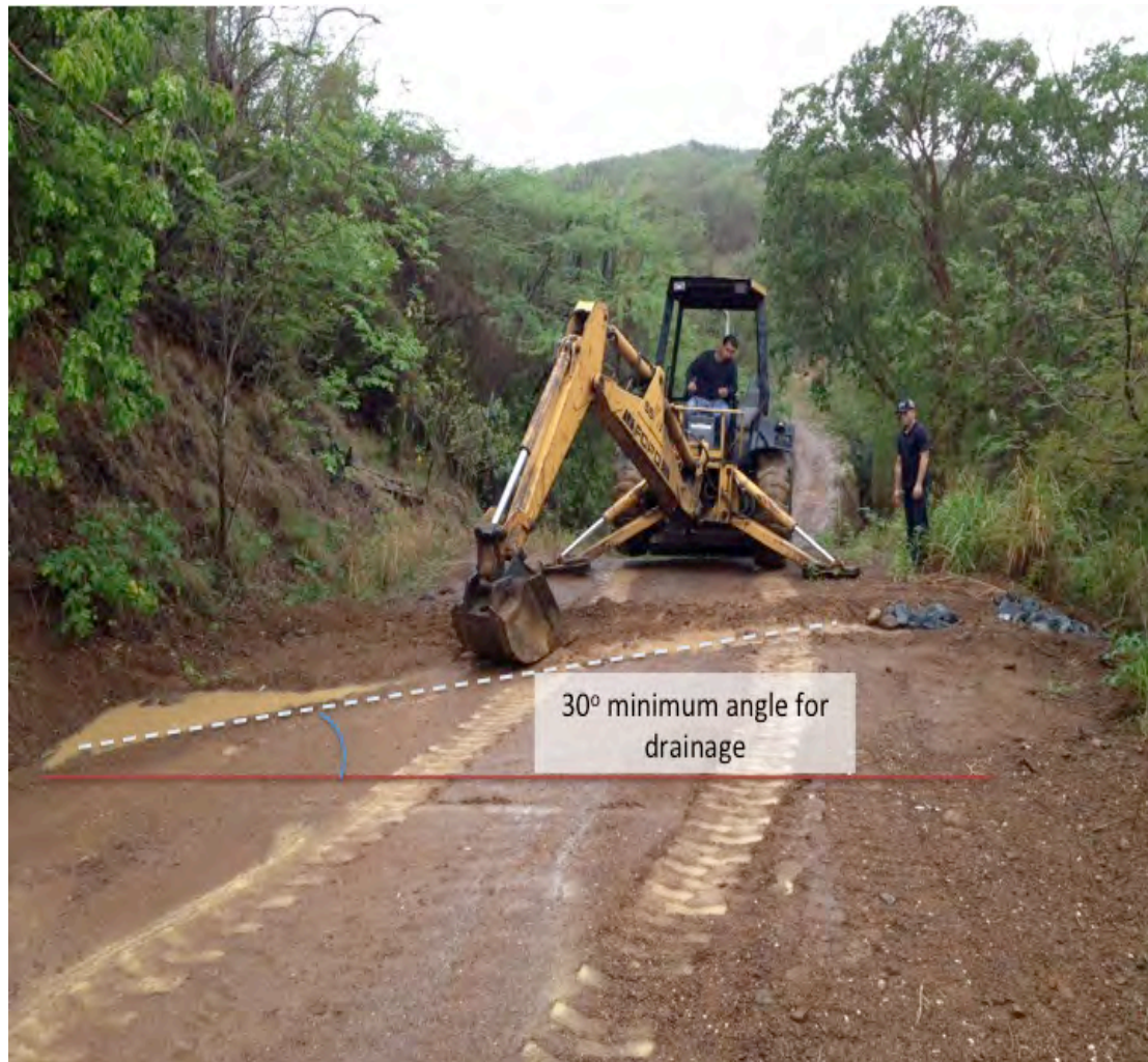
Figure 4. Example of a concrete or earthen water bar under construction in Culebra (based on NYSF, 2011)
