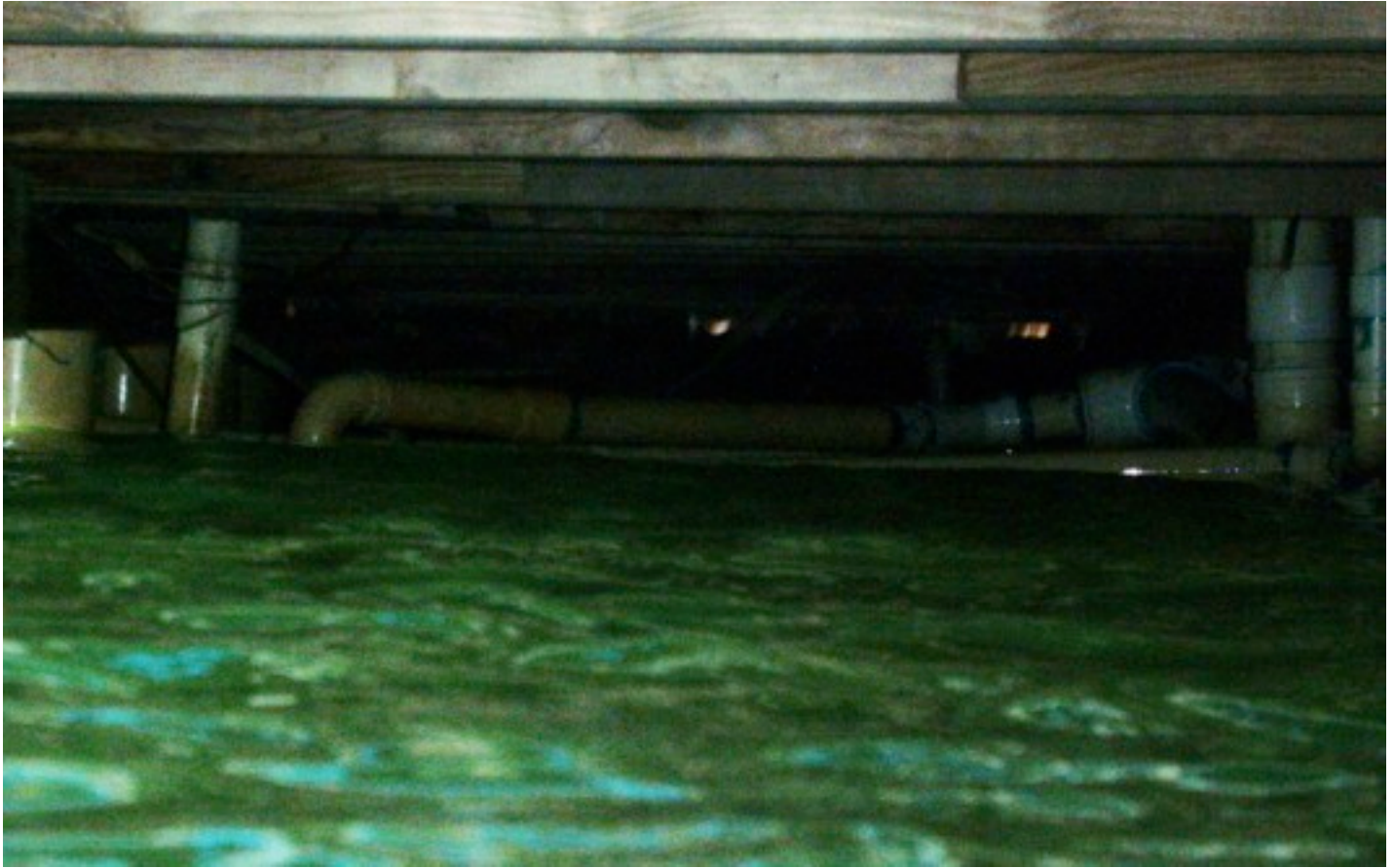
FIGURE 5: Residential PVC sewage profile with direct contact to seawater. We suspect that leakage can be occurring since there is no visible continuity.
