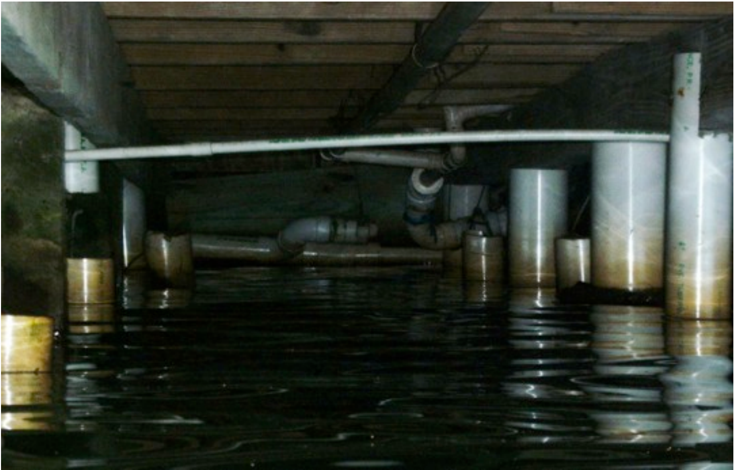
FIGURE 4: Residential PVC sewage profile. A common practice among most of the observed pipes is the use of loose caps. These may serve as a pressure breaker.
