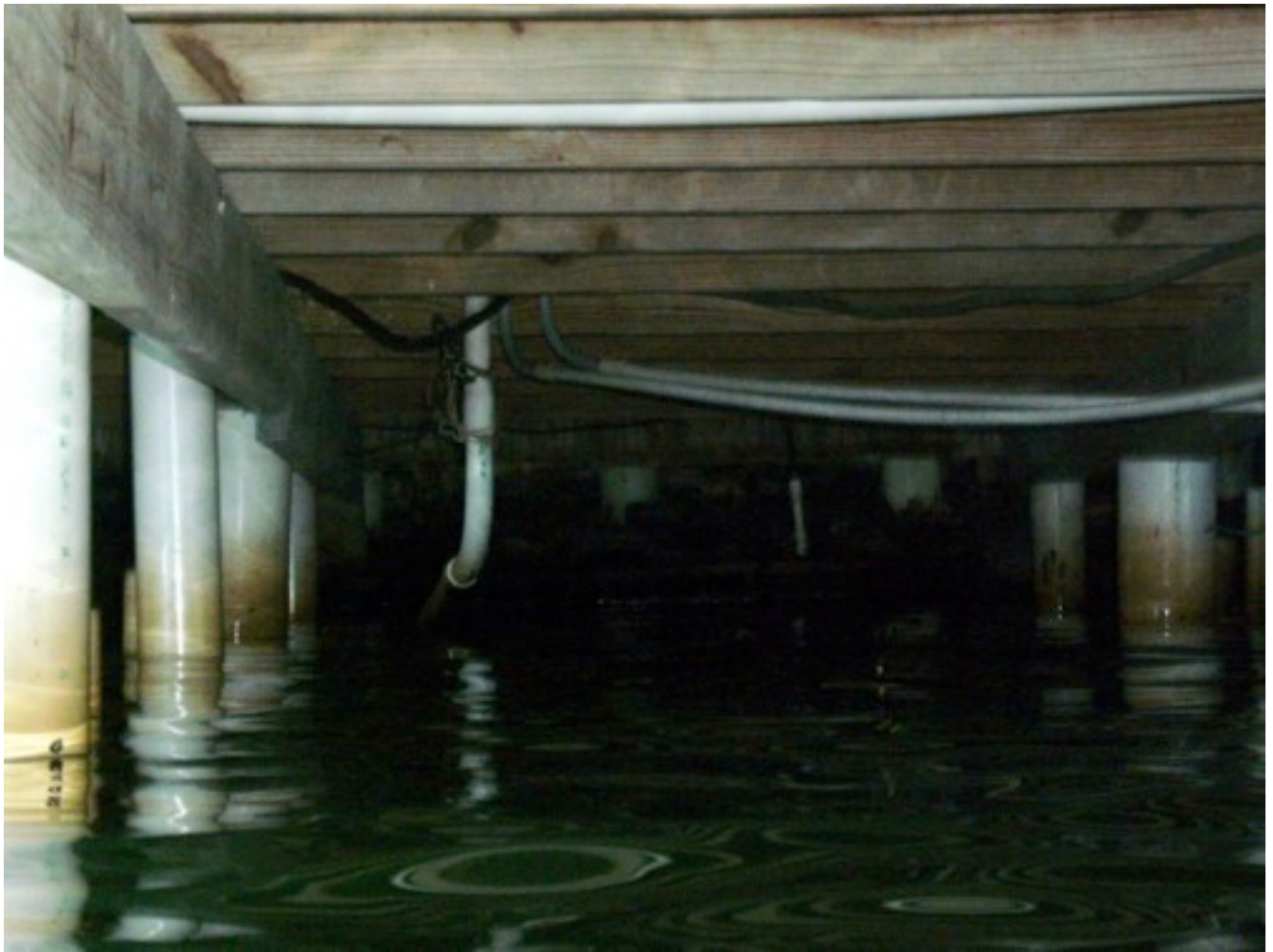
FIGURE 3: PVC pipe discharging directly into the water. This was a common finding among the stilt houses. Undesirable greases and detergents can enter the ecosystem. We observed surface greasy spots in the morning of the 8 th of February apparently from sinks and or boat cleaning activities.
