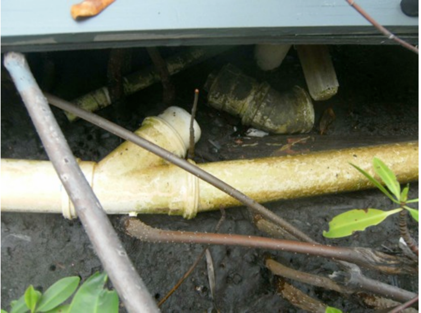
FIGURE 8: An open valve laying on its side (note discoloration) part of the sewage line near a stilt house entrance. These instances represent probable sources of contamination – certainly during heavy use and rain events if not general usage.
