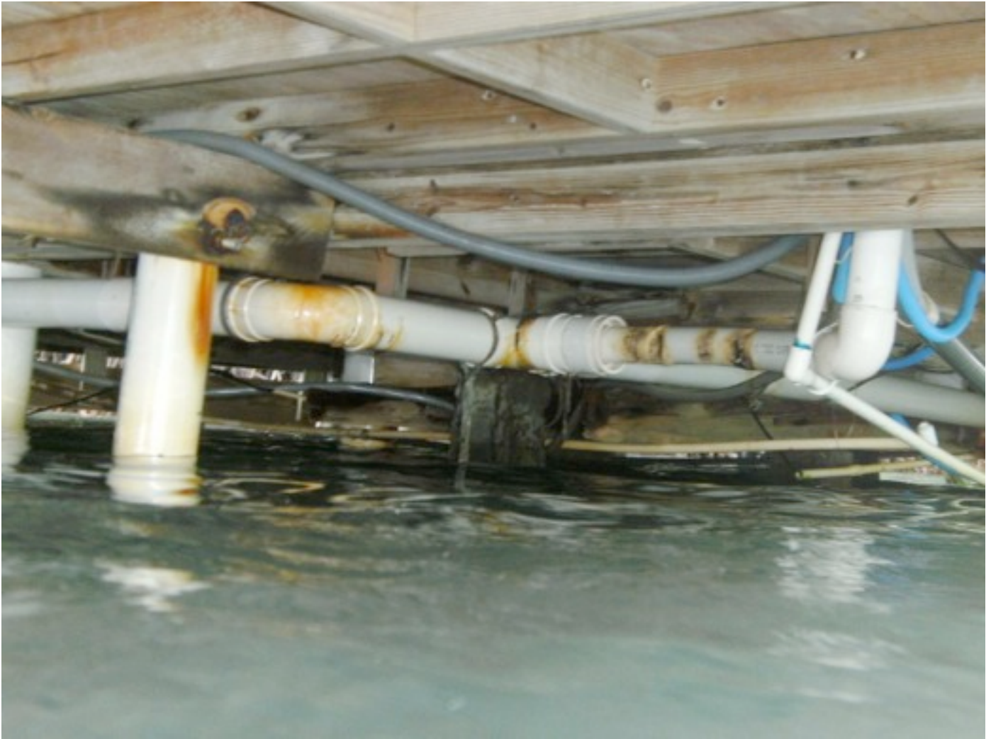
FIGURE 9: Residential sewer pipes with visible damages that can be leaching crude wastewater to the environment.
