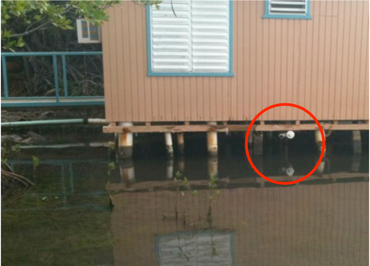
FIGURE 13: Note open pipe next to probable sewage end cap
