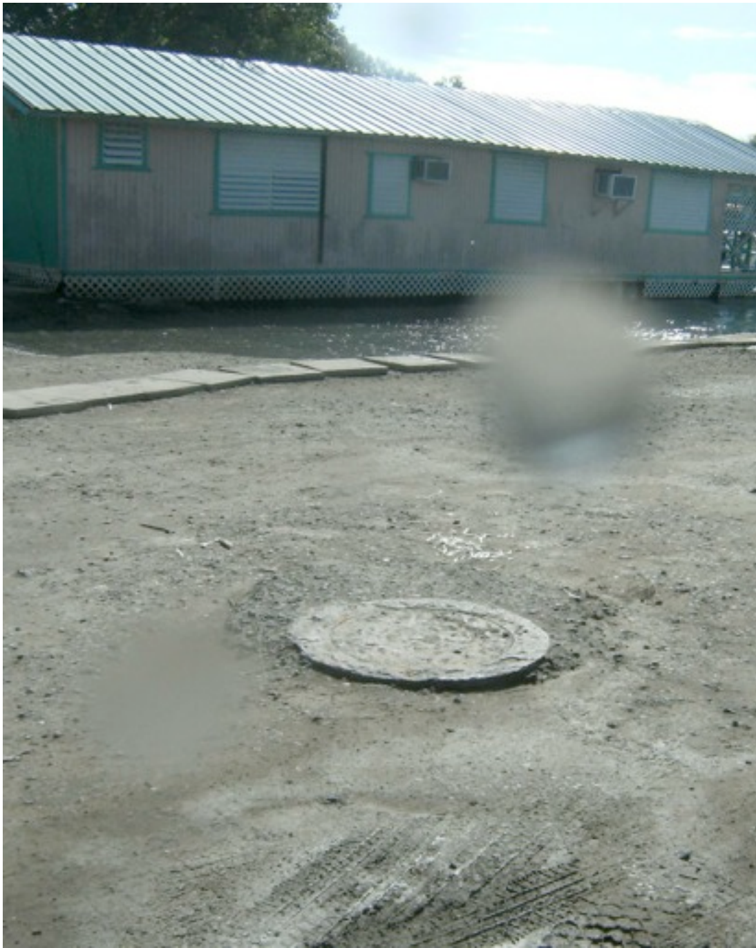
FIGURE 11: Manhole in front of UPR-Marine Sciences Laboratory. This manhole, when over flooded has been identified as a main contributor of raw sewage into the marine environment.
