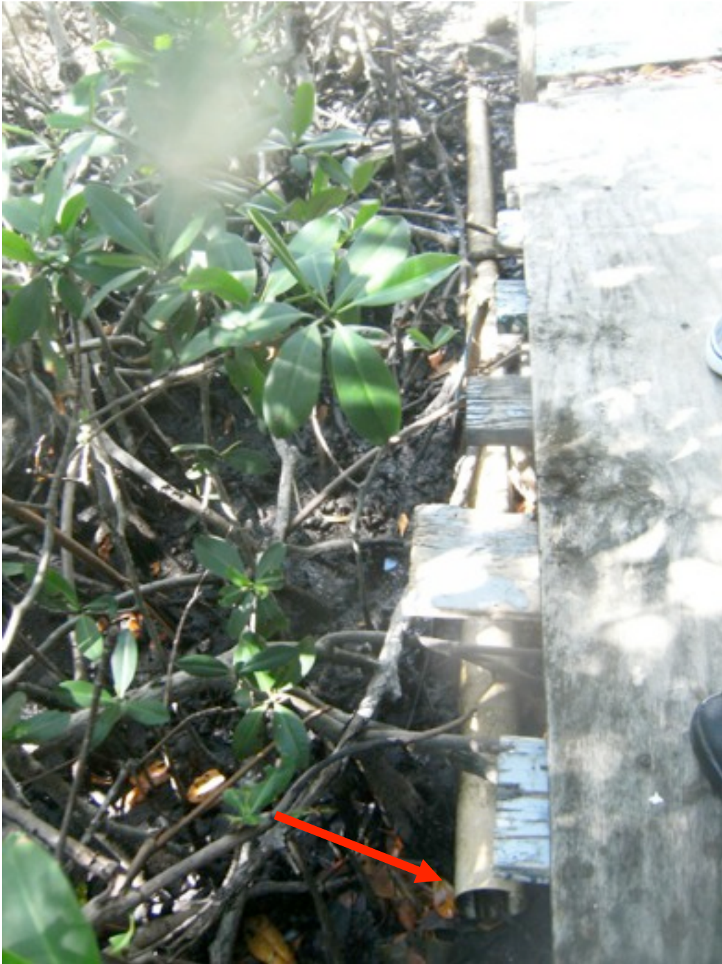
FIGURE 6: Where stilt houses were destroyed, the remaining residential sewage pipes can work as surcharge for the trunk main and as saltwater entrance to the sewer system which may interfere with the processes at the treatment plant.
