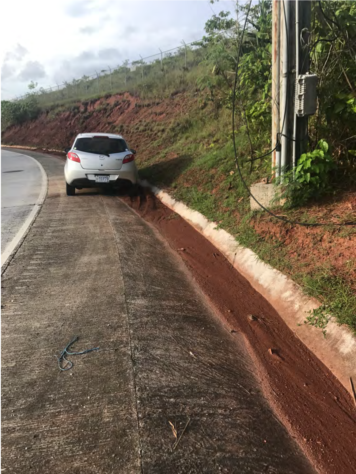
Figure 5. Eroding slopes adjacent to the Compact Road in Palau are a priority for stabilization
