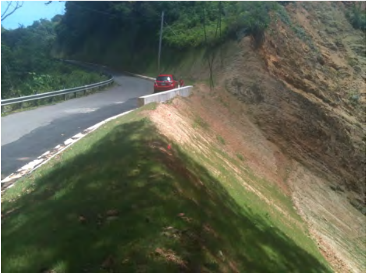
Figure 6. 7-23-12 Note Plot 3 with 50% vegetative cover and less vigorous grass growth was a thinner application of Flexterra (BFM) but also in an area with full sun and and high proportion of rock/consolidated material
